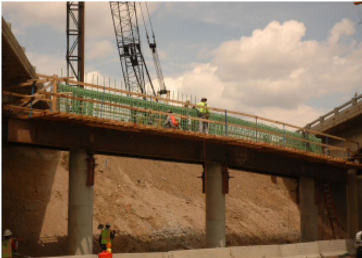
Construction of the new I-76 bridges over State Highway 224 and the Union Pacific Railroad is underway (Project #5)
