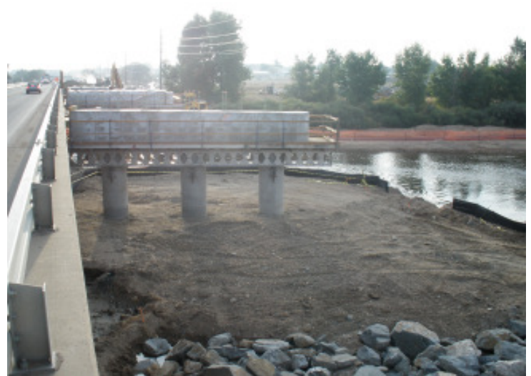
Construction of the new State Highway 7 bridge over the South Platte River is well underway. (Project #6).
