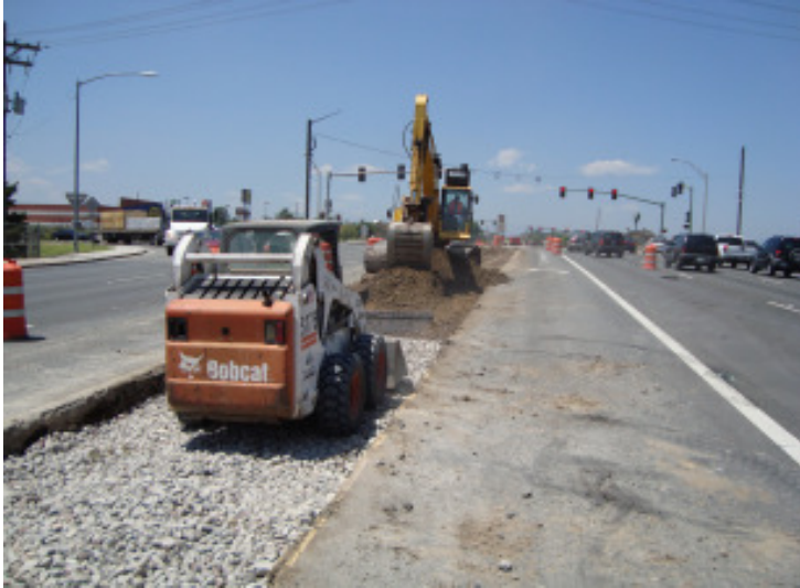
Crews prepare 104th Avenue for construction of the new bridge over I-25 (Project #2).
