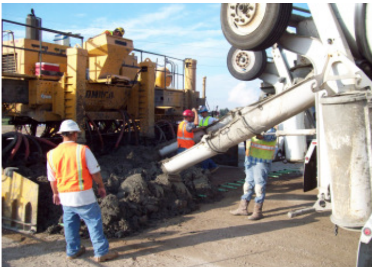
Crews pave the first half of the roundabouts on 96th Avenue at I-76 (Project #7).
