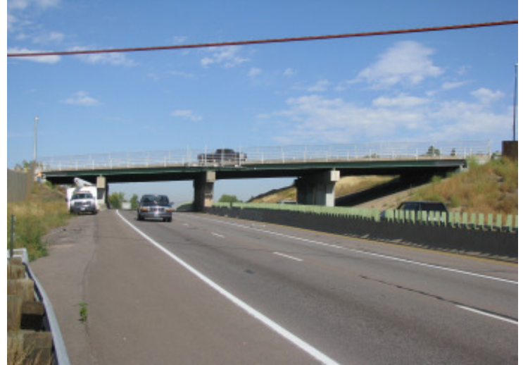
The existing 80th Avenue bridge over US 36 that was originally constructed in 1951 (Project #4).
