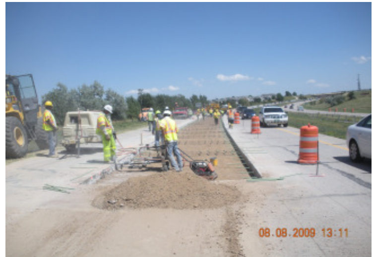
The concrete repairs on westbound C-470 are now complete, but work is still underway on eastbound C-470 (Project #24).
