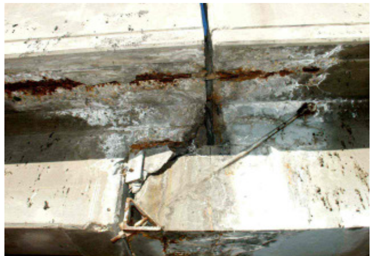
Condition of the current expansion joints on the I-70 viaduct (Project #10).
